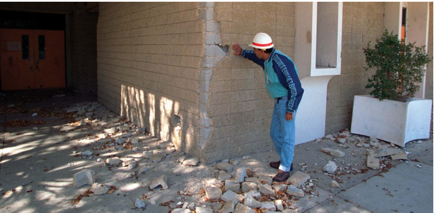
This photo, from the 1994 Northridge, Calif., USA, earthquake, illustrates that, while adequately designed buildings seldom collapse, earthquake damage to structural and architectural systems, and content damage, can result in significant losses. (Photo courtesy of FEMA)
