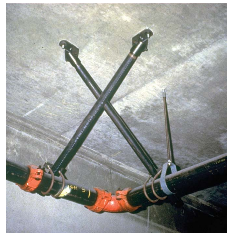
Proper earthquake bracing is essential, especially where piping changes directions.
