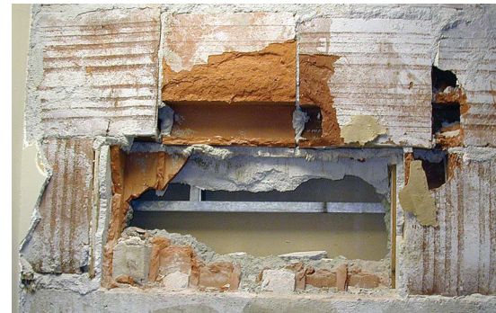
Hollow clay tile partitions (e.g. surrounding stairwells) always perform poorly in earthquakes and should be avoided, even in low seismicity areas.
