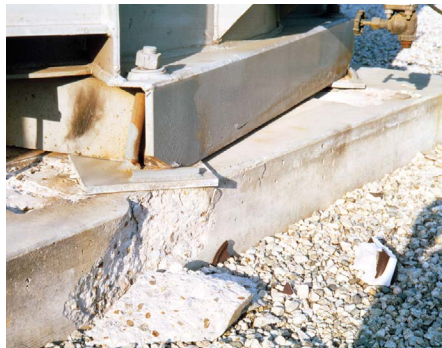
Inadequately designed or installed equipment anchorage may not prevent movement in very severe ground shaking.
